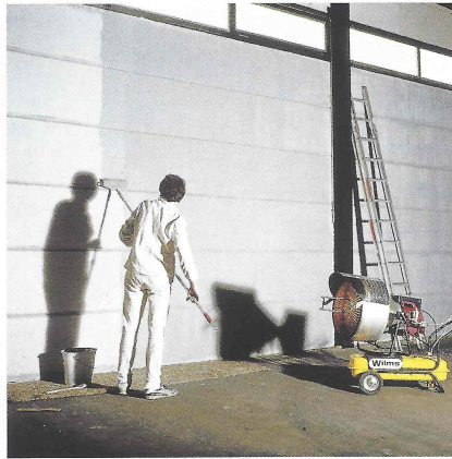
Heating and drying on constructions sites
